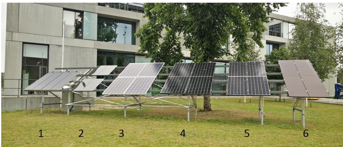
Figure 1.1: The set-up of the installed solar panels at AMOLF. The panels face South and are located next to a tree. In order from panel 1 – 6: CIGS, CdTe, Poly-Si, IBC Si, HIT Si and CIGSm.
